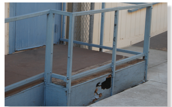
Wood with extensive termite damage needs to be replaced.
