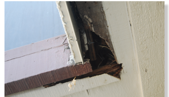
Deteriorating roofs at local schools are in need of repair.
